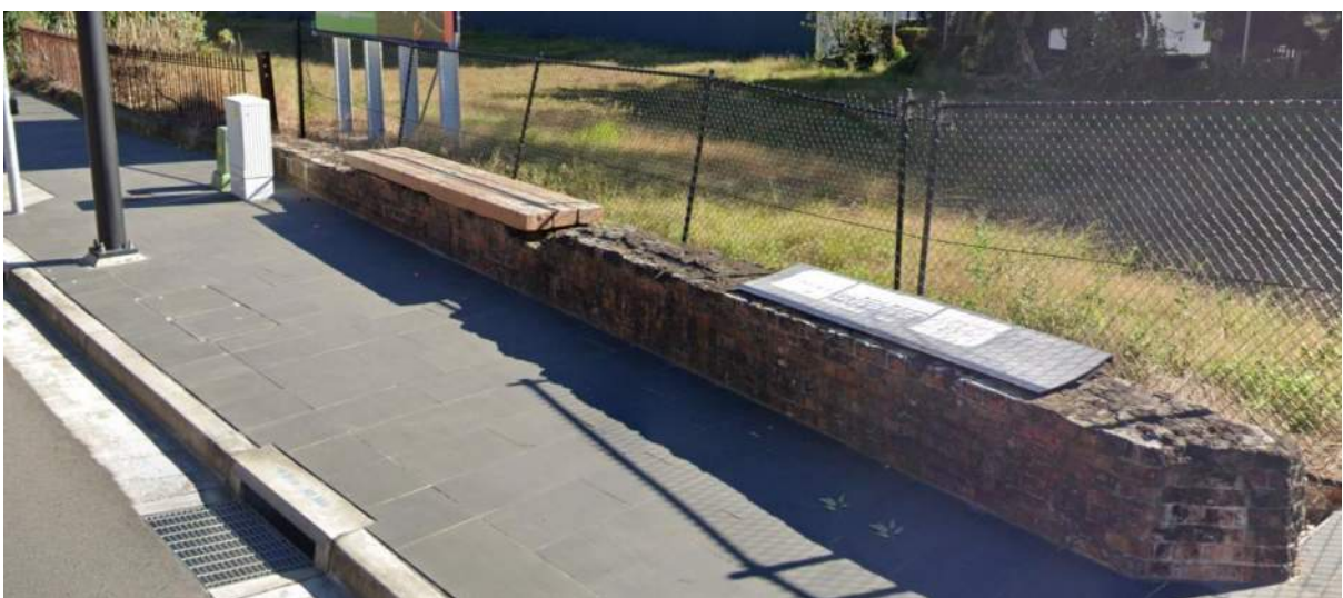
Figure 88: remains of AA Company Bridge and Fence at 280 Hunter Street (Source: Google Streetview)
