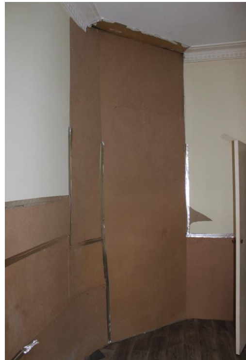
Figure 40: MDF board installed to cover the location of the former fire place in the western front room.
