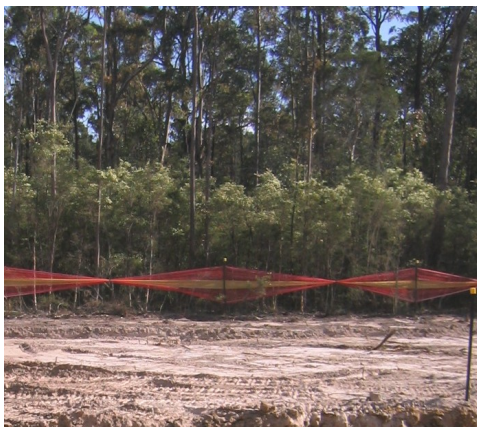
Barriers can be used to mark vegetated areas as 'no go' areas.
