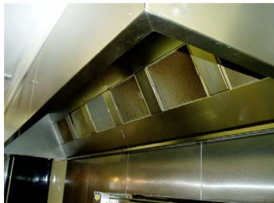
Picture 2: Mechanical exhaust system.
