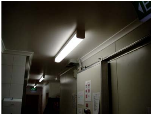
Picture 3: Light fitting with diffuser cover
