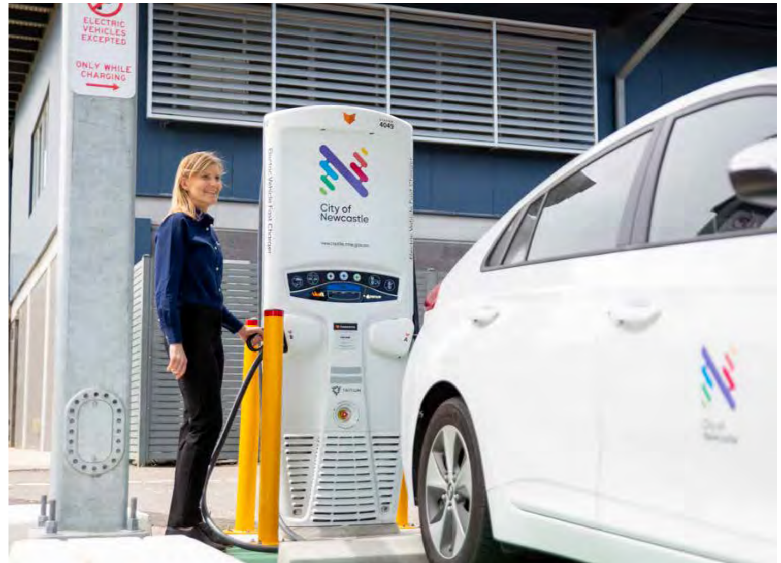
EV Charging Station.
