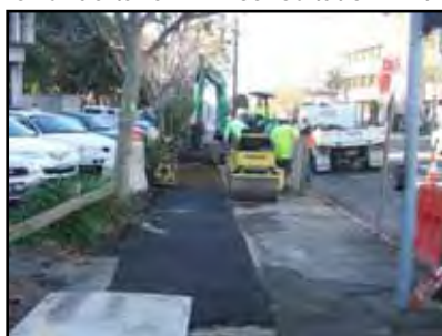
Utility works often damage public
