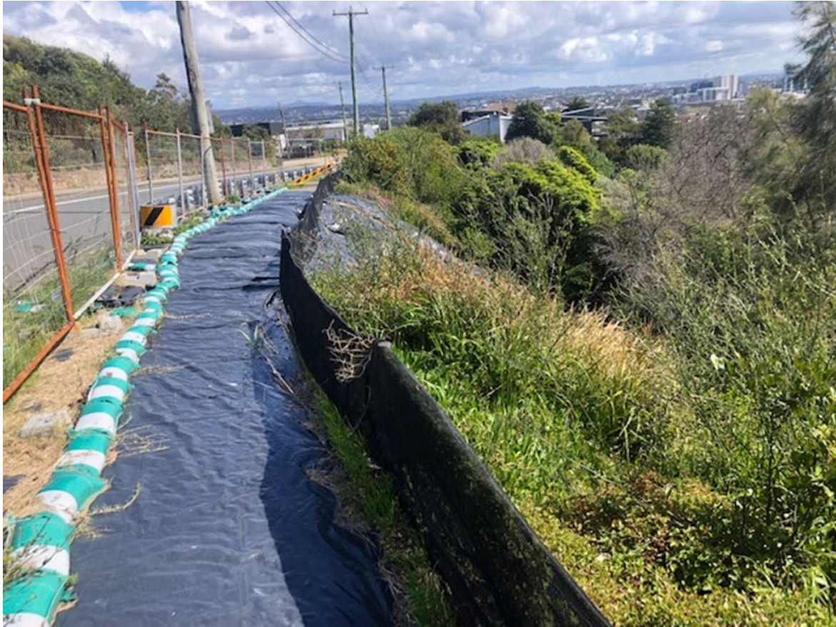
Plate 1 Top of Memorial Drive looking west with temporary slope stabilisation measures
