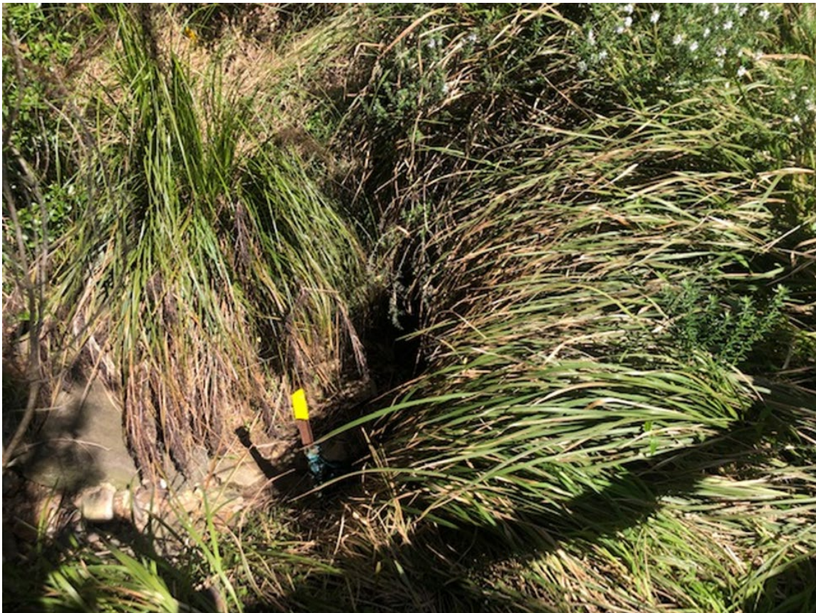
Plate 8 Existing inlet to pit and pipe stormwater system which conveys water across Nesca Parade into Nesca Park
