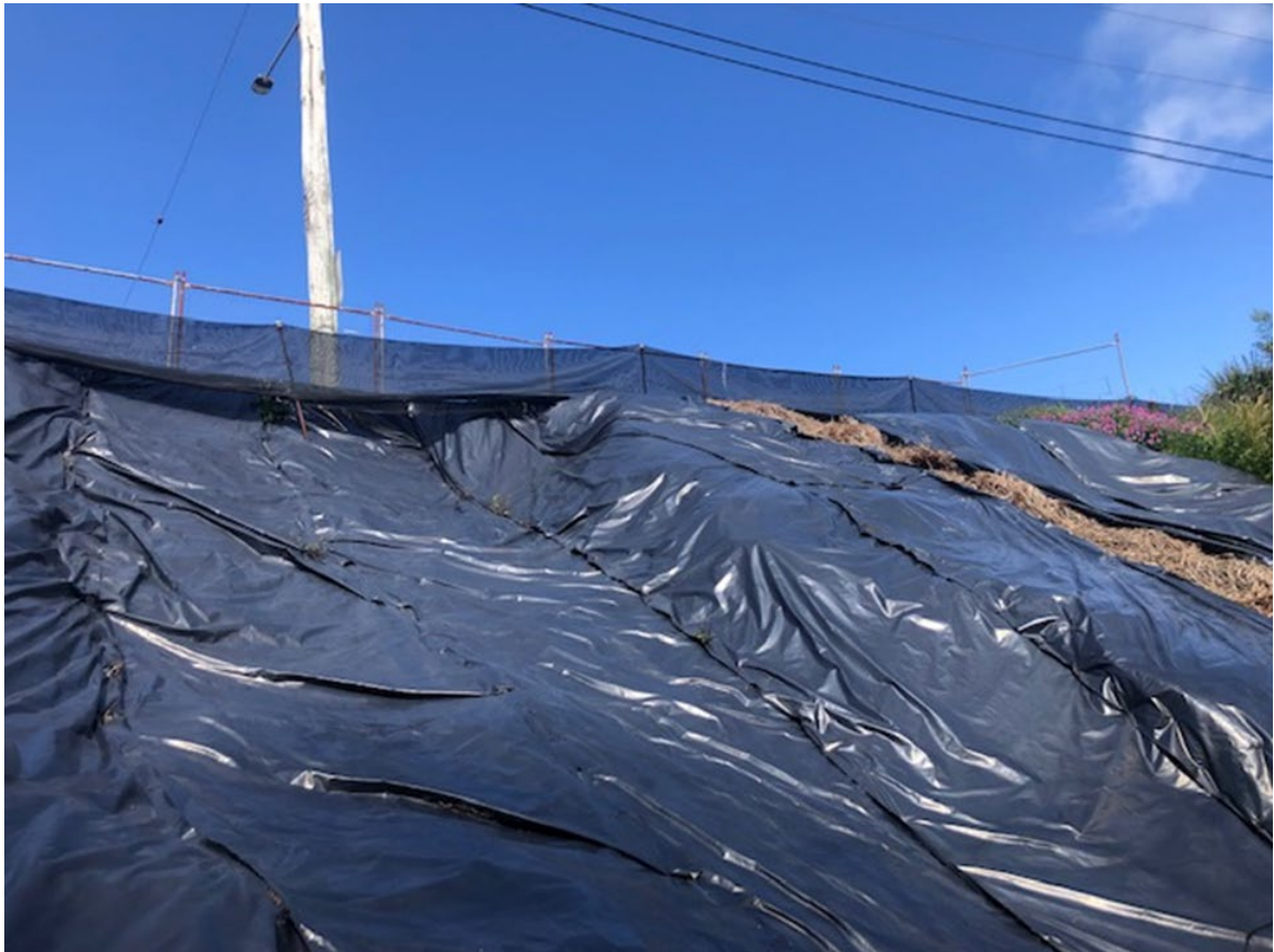
Plate 4 Area where stabilisation and remediation will occur, looking south towards Memorial Drive
