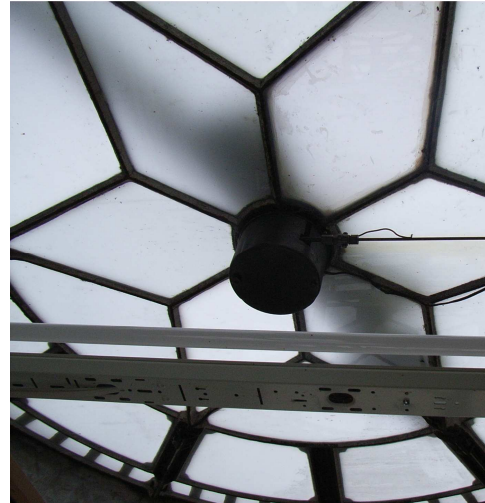
Figure 24: Inside face of the NCH Clock 2008
