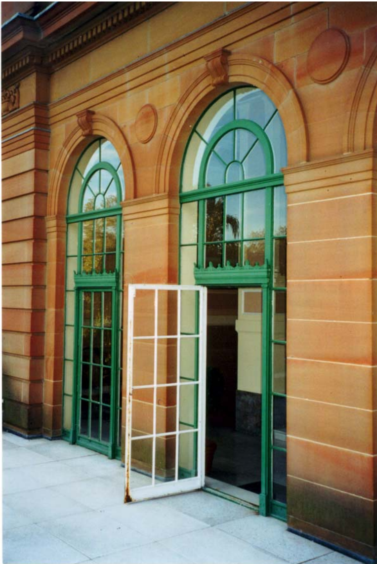
Figure 6: View of the steel doors opening onto the Balcony above the porte cochere (Photo 2001)
