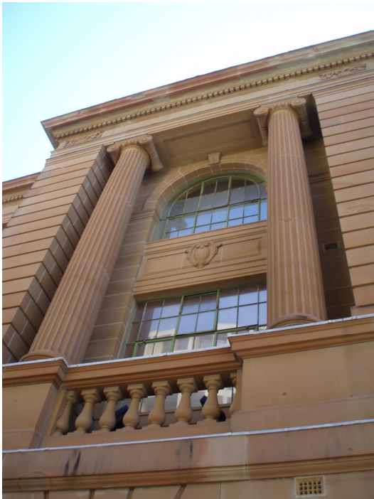
Figure 30: Façade Detail 2007 showing recessed façade areas. The sandstone is in better condition in these areas however the balconies formed at the base of the recesses have drainage problems.
