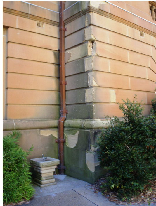
Figure 31: Façade Detail 2007 showing deterioration of sandstone due to failure of sandstone steel fixings and past failure of rainwater system. Landscaping around the perimeter of NCH also needs review.
