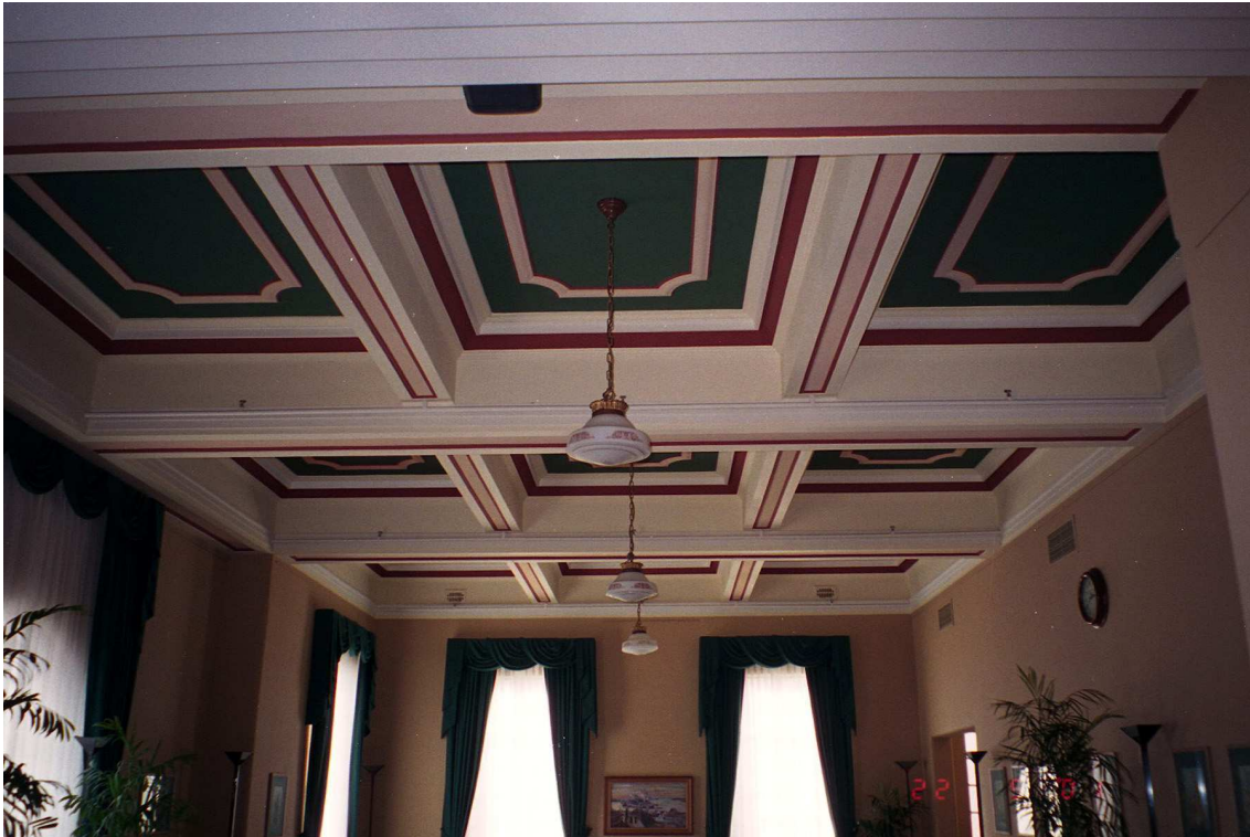
Figure 22: Ceiling Detail 2001 showing 1980s colour scheme. Original decorative schemes were more restrained in such spaces.
